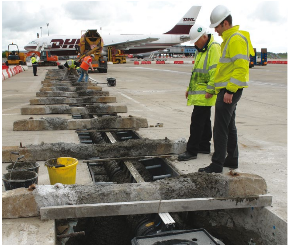
ACO Qmax 600 and 900 used in the cargo area of the apron.
