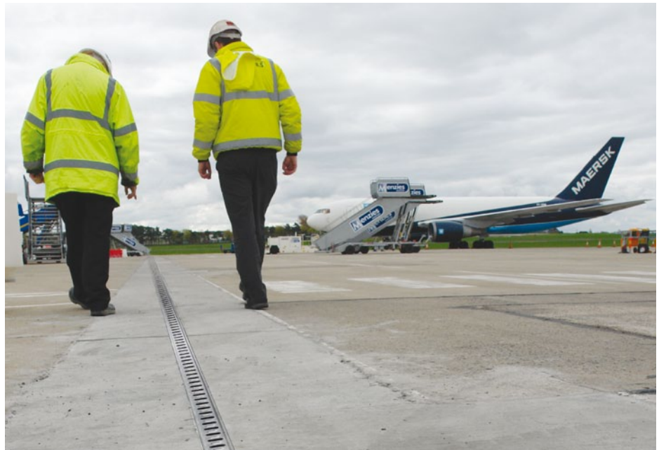
ACO Qmax 225 and 350 used on the upgrade to the existing west apron.
